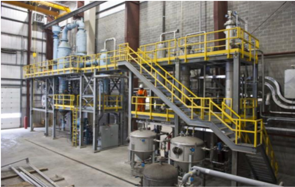
Figure 16: Enerkem's WTFC pilot facility in Edmonton
